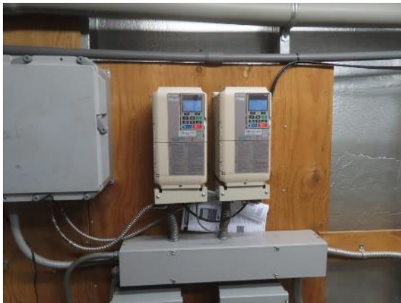
Well House #1 Relays
