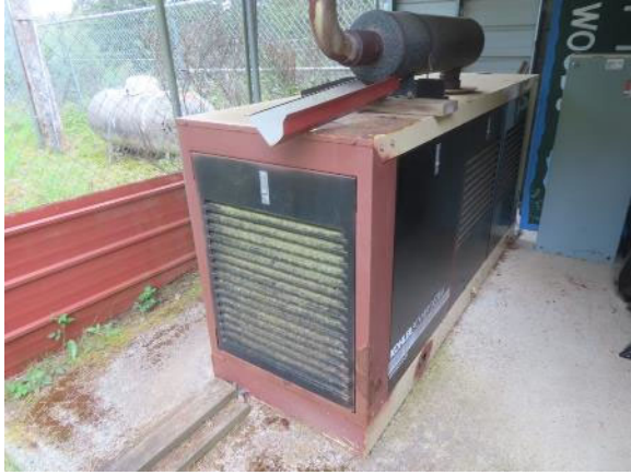
Electrical Generator at Well House #1
