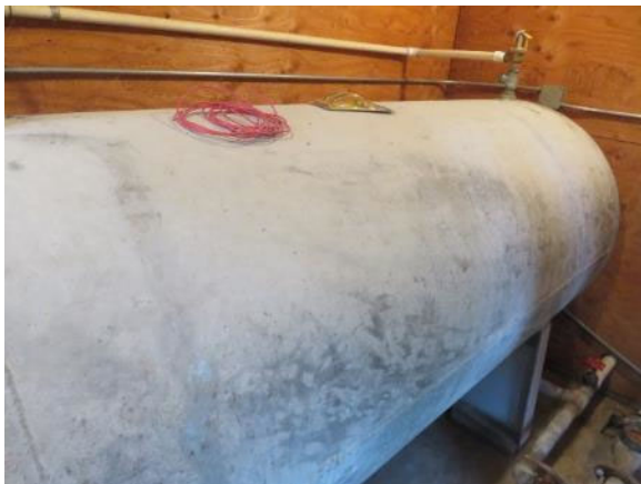
Metal Storage Tank at Well House #4
