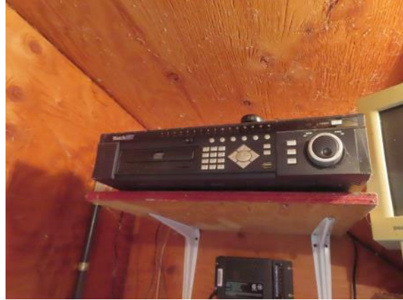
Surveillance System Recording Equipment
