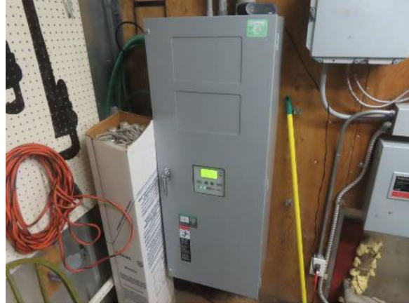
Transfer Switch for Electrical Generator at Well House #1
