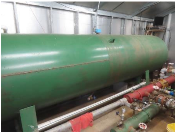
Metal Storage Tank inside Well House #4
