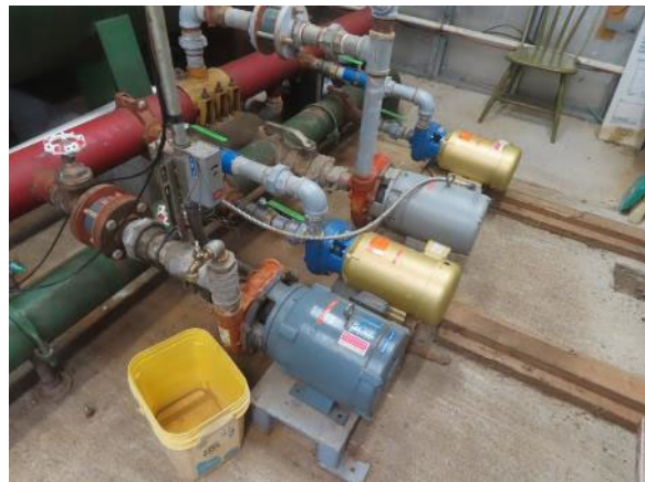
4 Booster Pumps (of which 2 are older back-ups)
